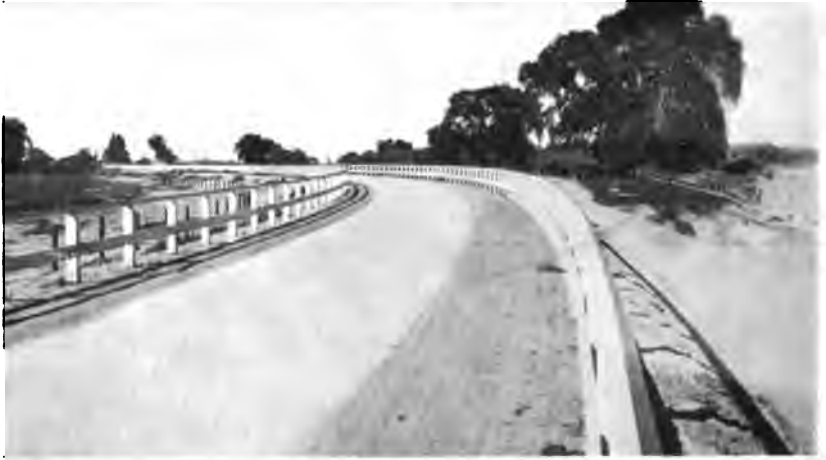
Adobe fill on Modesto-Crows Landing road.
